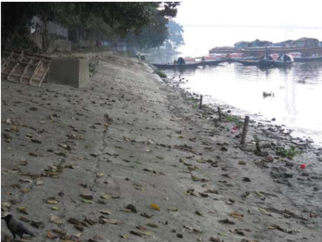
Plate 204 – Condition of Embankment near Outram Ghat
