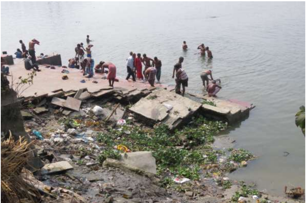
Plate 198 – Condition of Embankment near Jagannath Ghat
