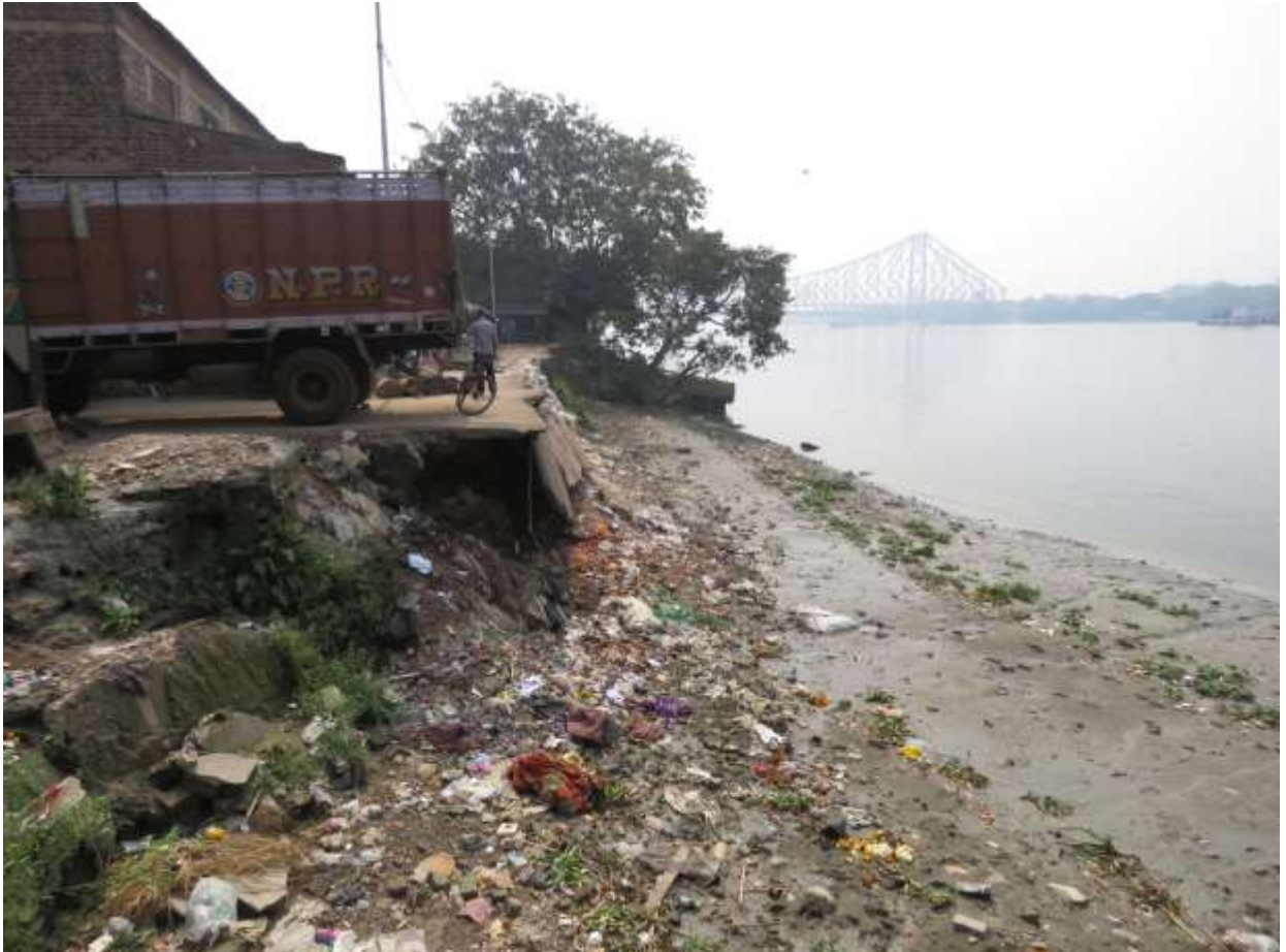
Plate 195 – Condition of Embankment, in between Nimtala Ghat and P.KTagore Ghat .
