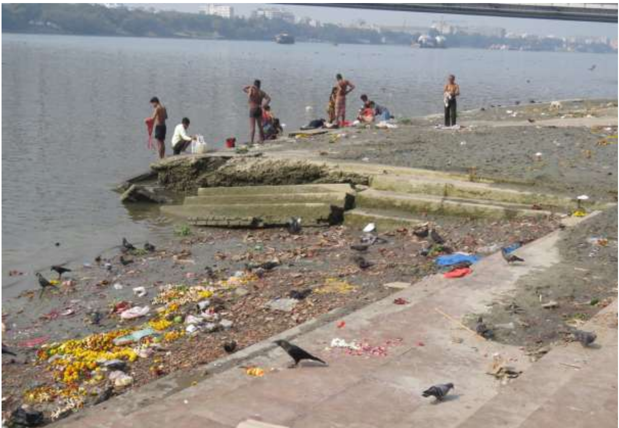
Plate 200 – Condition of Embankment, Chhote Lal ki Ghat
