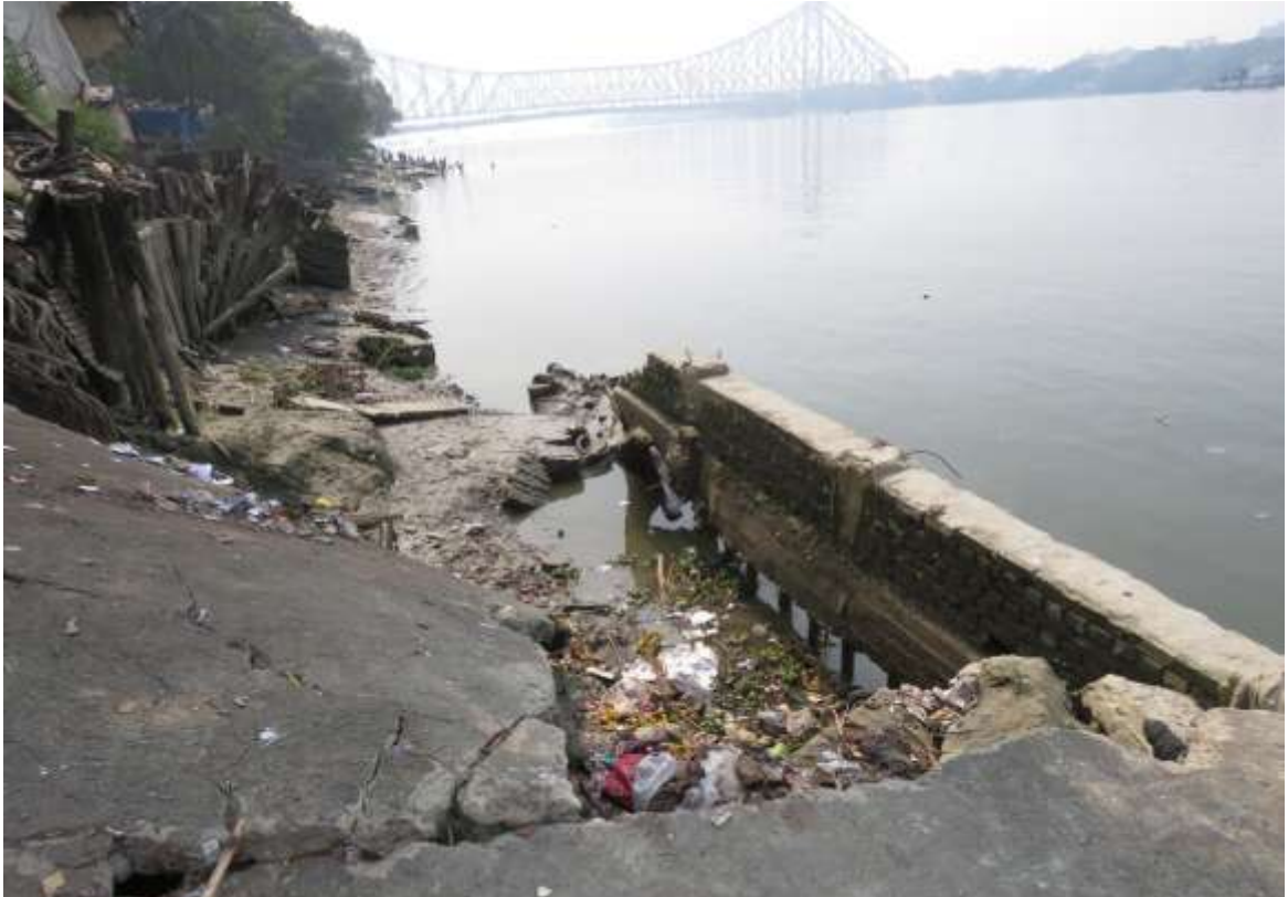
Plate 197 – Condition of Embankment near P.K Thakur Ghat
