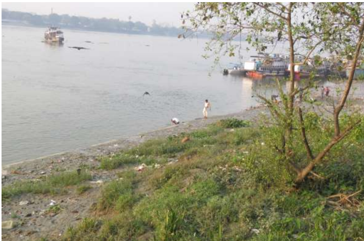
Plate 202 – Condition of Embankment near Fairlie Jetty
