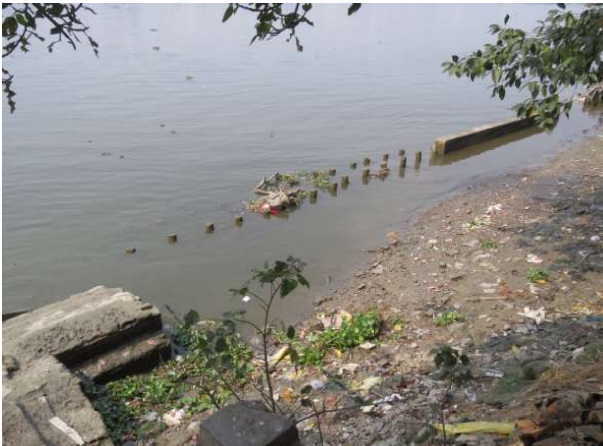
Plate 196– Condition of Embankment near Prassana Kumar Ghat
