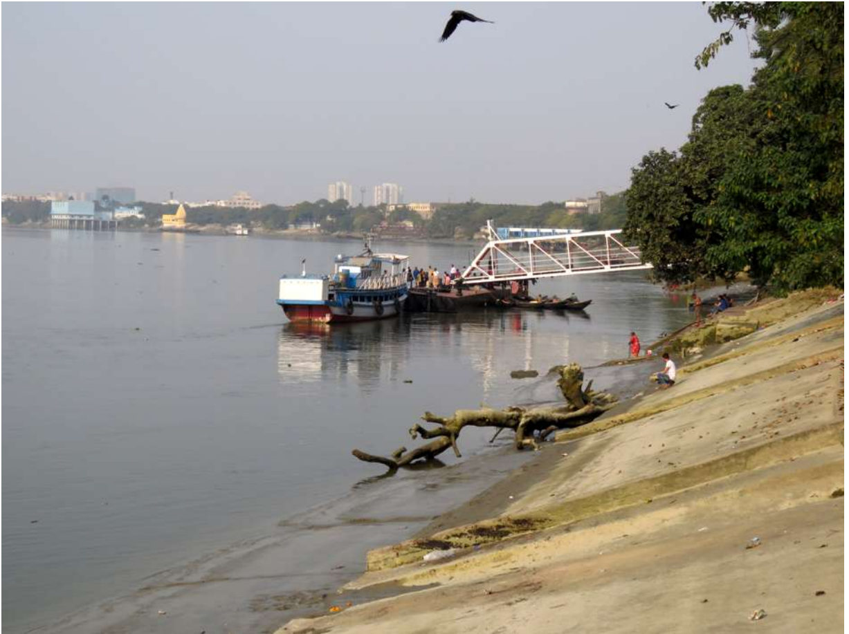
Plate 190– Condition of Embankment near Sovabazaar Ferry Ghat
