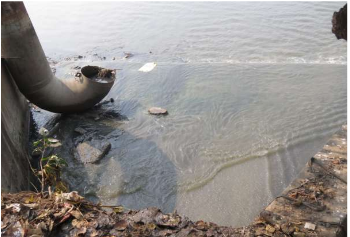
Plate 214: Sewage Outfall near Barabazar
